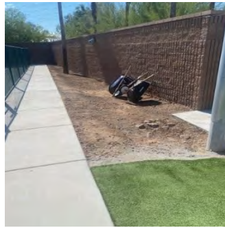
Removed rocks west of Court 20 in preparation for contractor to grade & install artificial turf on September 25
